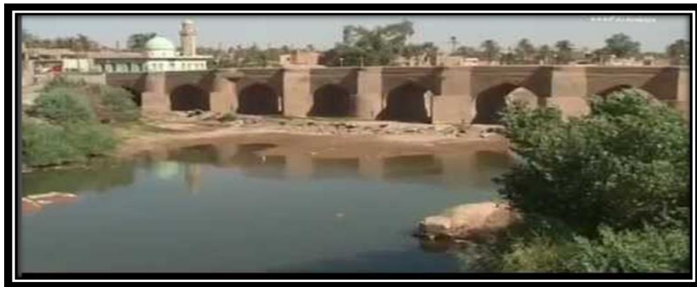
Figure 3. Al-Wand Dam, which was built on the Al-Wand River Field study in 5 -2- 2021
